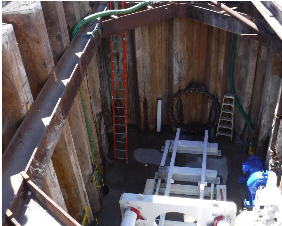
This shaft was Contractor-designed – the sheetpile, the walers, and the entry ring.
