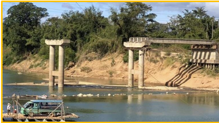
Precast beams in Laos (after a washout).
