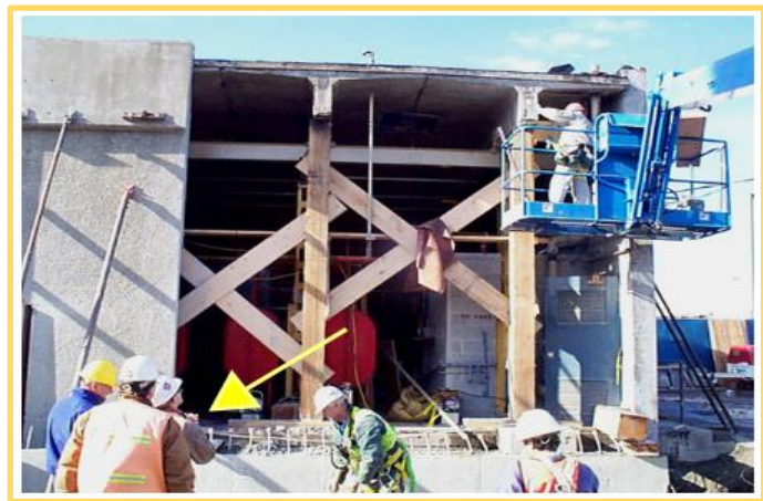
This photo is called "Praying Man." Me in 2001 at age 30 as the project manager, praying that we could hold this roof over top Seatac International Airport's domestic/fire water pump station while we reconstructed its guts and this wall. This shoring system went through an earthquake!
