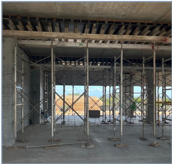
Shoring towers/frames with metal beams and plywood above forming the underside of a beam or floor.
