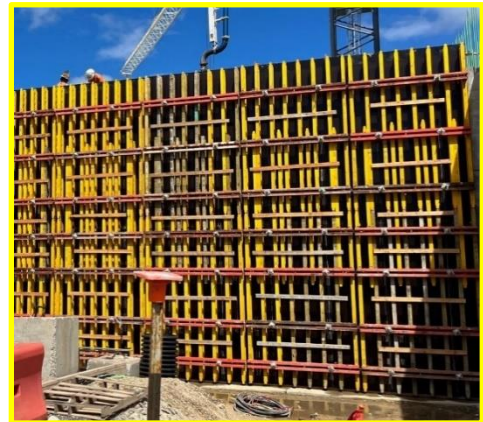
Concrete being poured into wall formwork. This is a gangwall because the form is so big and it was formed on the ground and flown in with the crane (versus a smaller wall which may be built in place).
