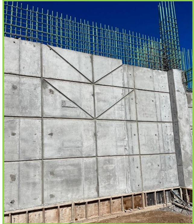
Notice the architectural feature in this wall. This is usually formed with chamfer or a form liner.
